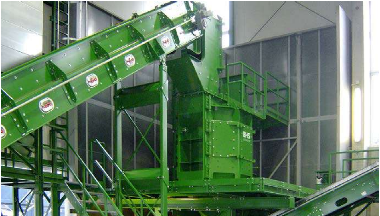
Installation of a complete BHS recycling plant for crushing secondary metals in Austria. The plant is centered on a Rotorshredder from BHS, shown here without its final sound-proof enclosure.
