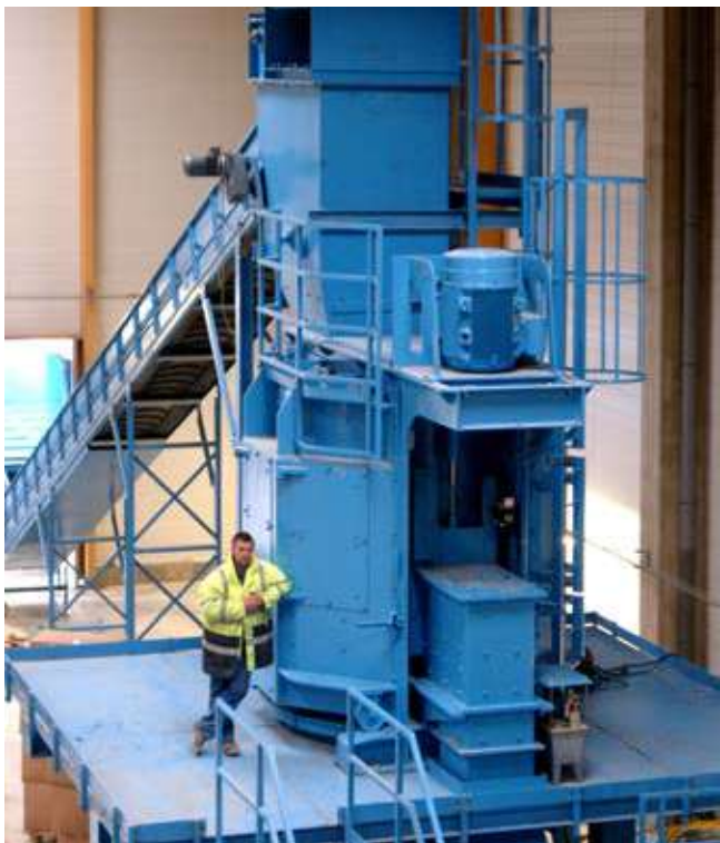
Construction and assembly of a complete BHS recycling plant in France. The E-Scrap plant is equipped with a BHS Rotorshredder of type RS 2018.
