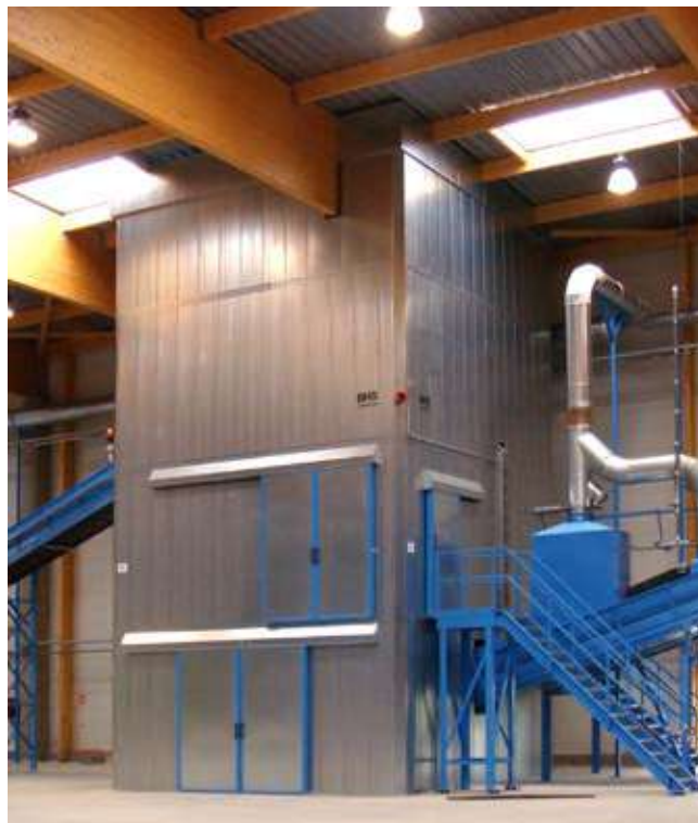
The Rotorshredder is enclosed for disaggregation of E-Scrap in the first recycling stage.
