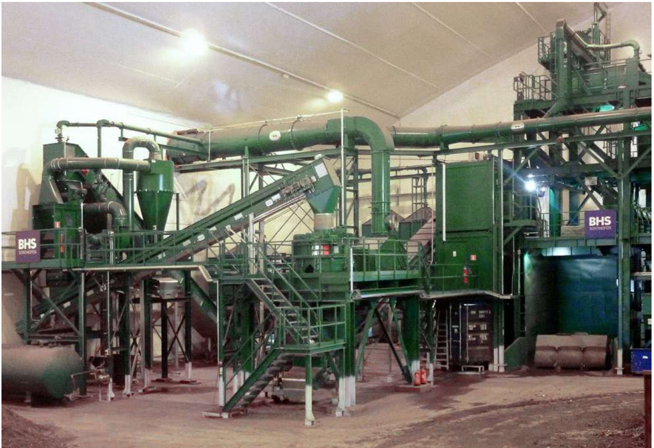
Recycling plant for the fine preparation of shredder residue fractions with RPMV 1513 in Finland
