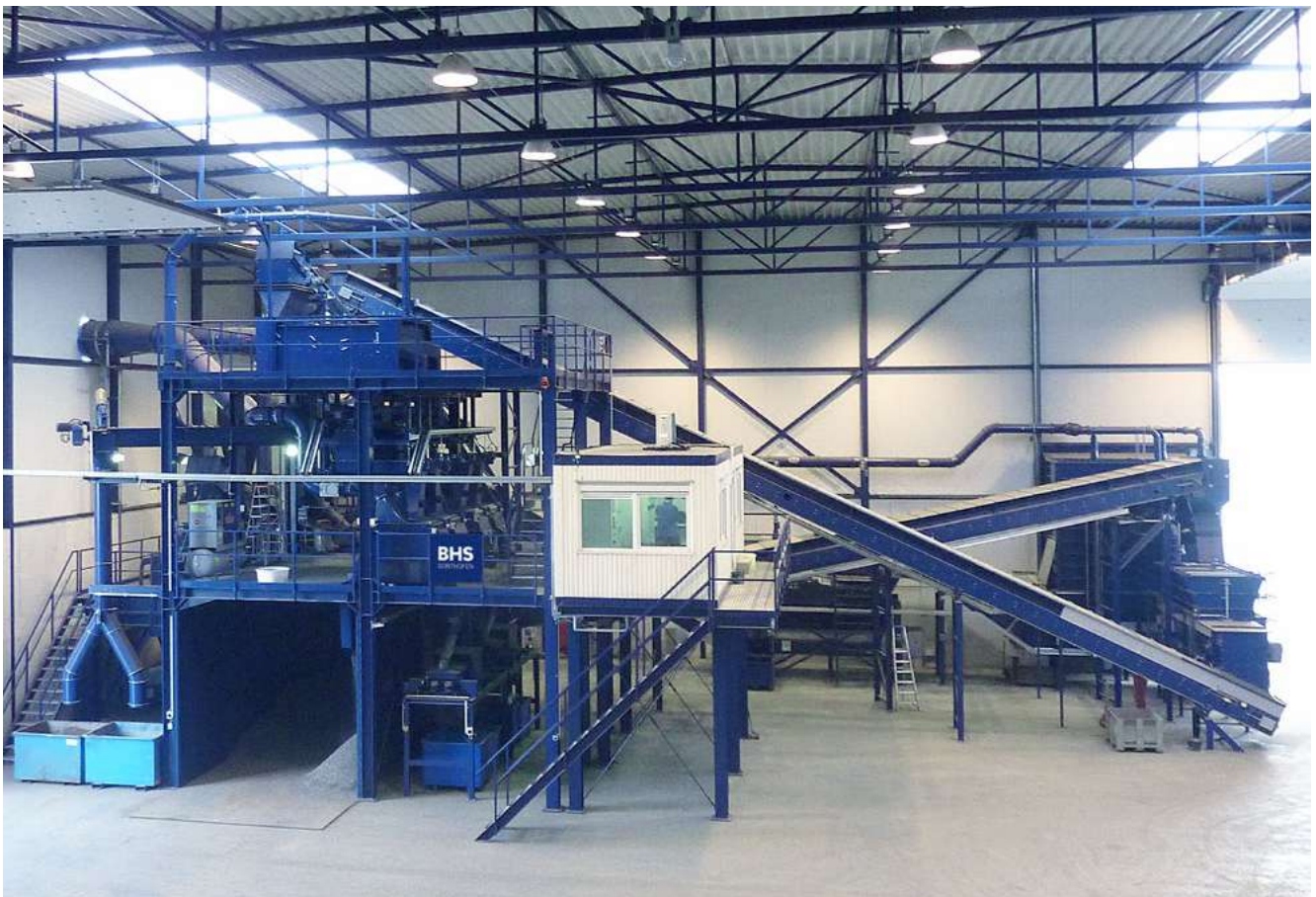
Recycling plant for the fine preparation of shredder residue fractions with RPMV 1513 in Holland
