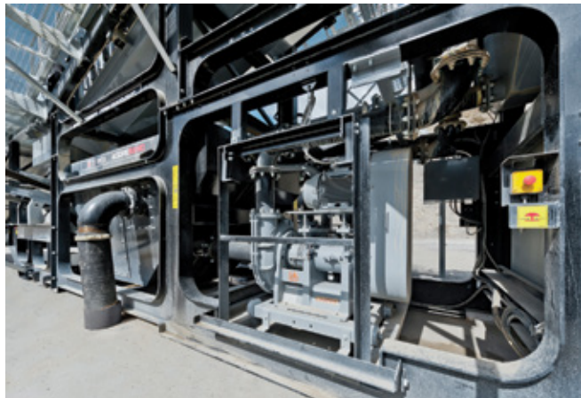
Centrifugal Pumps, Roll out for Service Access
